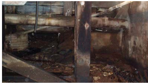
The unprotected timber piles that received marine borer damages.
