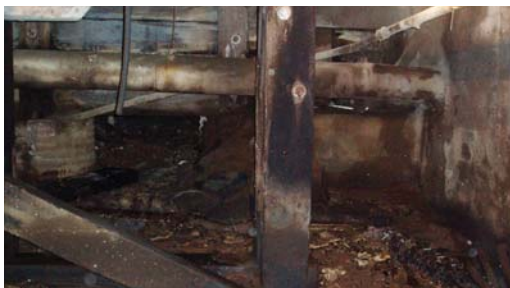
The unprotected timber piles that received marine borer damages.
