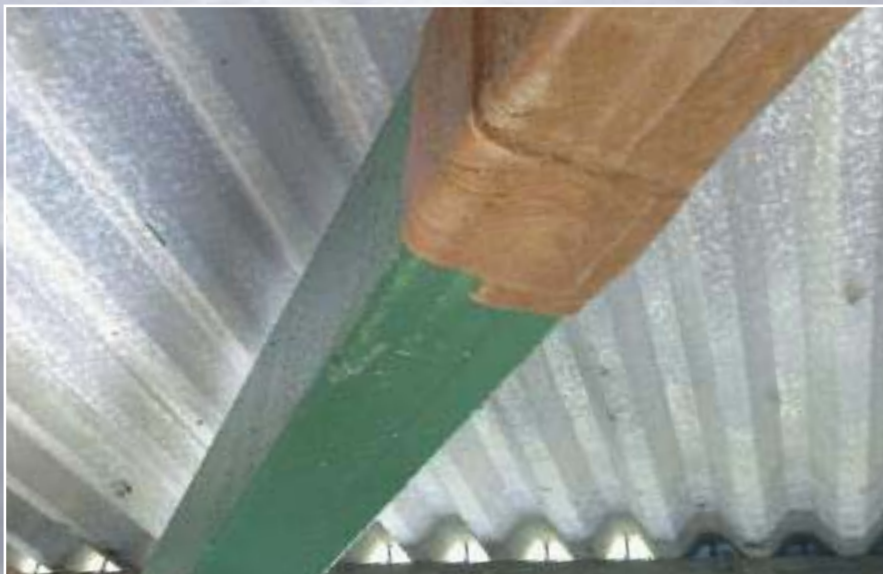
A Denso Petrolatum Tape system was used on steelwork in the conveyor tunnels
