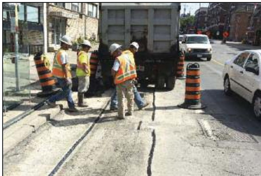
The Densoband in place along both of the vertical joint faces of the reinstatement trench.
